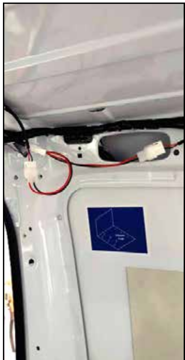
Step 34 BW1 makes connection to LEDR and LEDL at this location, immediately behind center top roof rib.
